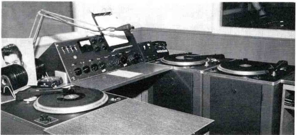
FIG. 3. Typical installation of several BQ-2C's gives a custom look to the studio.
